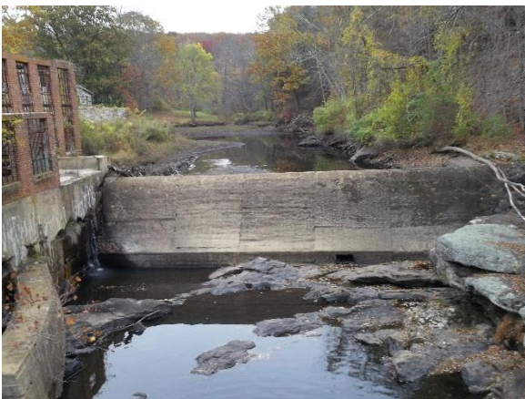
Norton Mill Dam prior to removal with the ruins of the old paper mill to the left. The dam was so leaky that during low flows of summer, it didn't maintain the pond, which can be seen behind the dam, drawn down. Note the rock outcrop along the right side of the photo.
