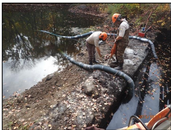
The pond behind Straight Pond Dam was drawn down using siphons (long black hoses) and then the jackhammering began.
