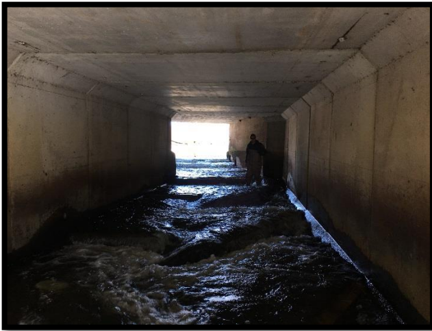
The Clark's Pond Fishway on Indian River in Milford has two sections. The lower section, shown above, consists of off-set baffles in a sloped box culvert. Our crew replaced rotting timber baffles last summer with concrete. Upstream is a pool-and-weir fishway spanning a drop structure.
